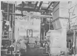
First of three Tosi Boilers completed.
